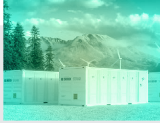
Battery Energy Storage Systems
